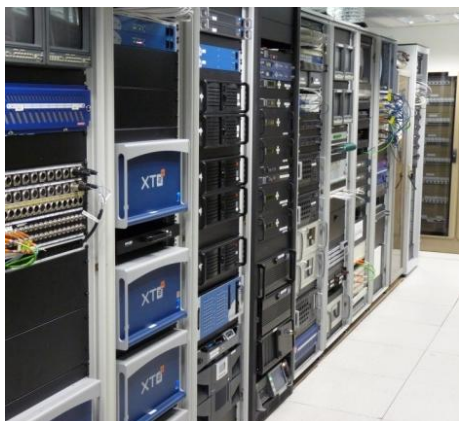
The main Technical Room
